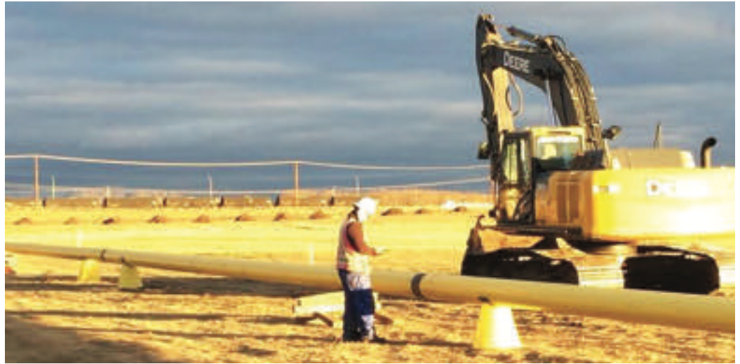
Lance Fugate of Enmapp inspects pipeline construction using the Arrow 100, TerraGo Edge on iPad in Canada.
