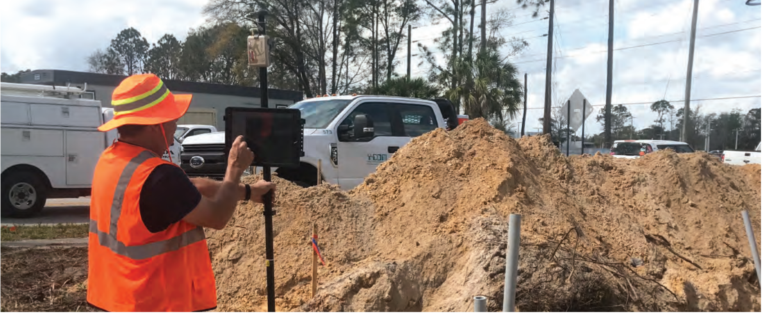
A NSBU mobile worker collects assets using ArcGIS® apps on iPad® with an Eos Arrow Gold® GNSS receiver on a rangepole.
